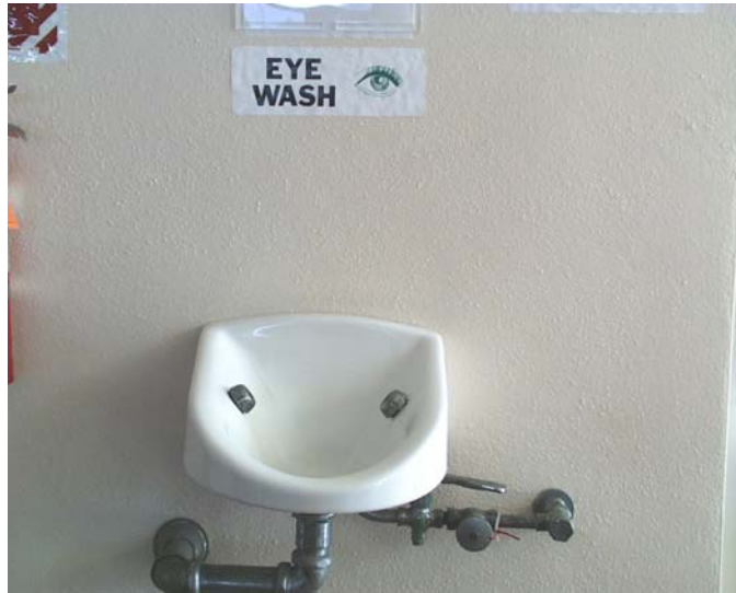
Emergency Eye Wash Station
